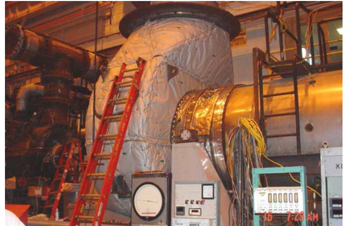
Gas Turbine Exhaust Housing
