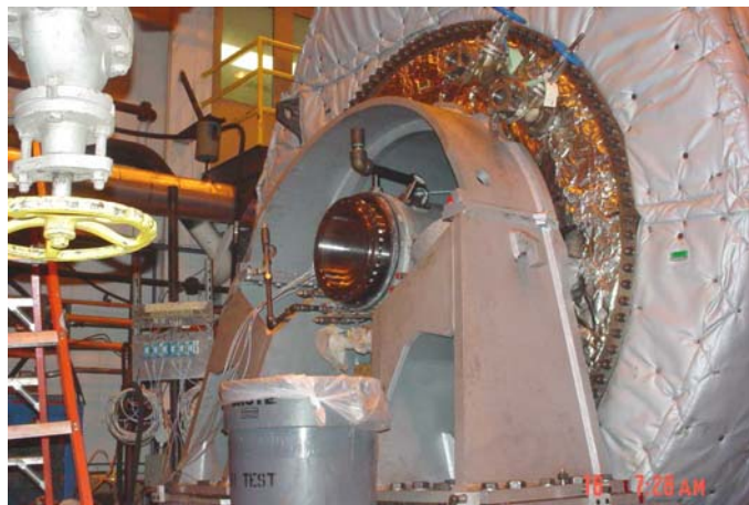
Gas Turbine Exhaust Housing
