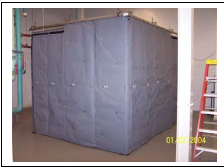
Acoustic Enclosure – 15 DBA Reduction
