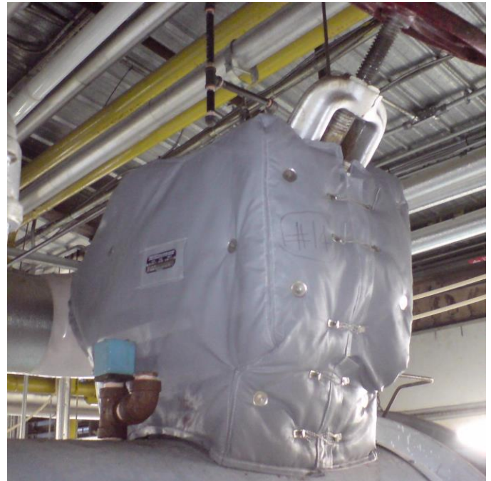
Main Boiler Stop-check Valve
