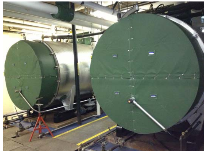
243 CM Diameter - Boiler Doors
