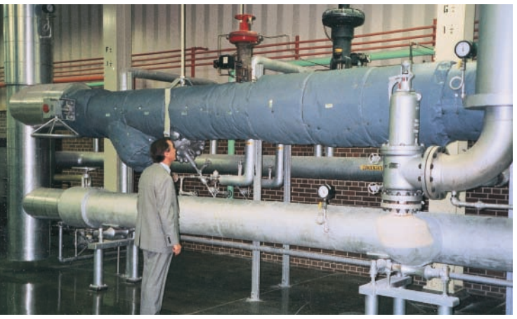
20" STEAM INLET - PRV STATION Design: LT450A-TT - 2" thick
